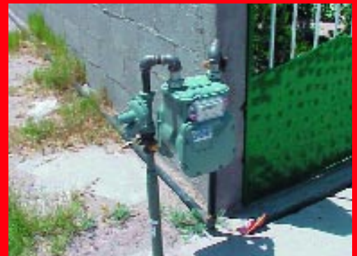
Residential installation in Ciudad Juárez – American Meter CR4000 regulator and AC-250 meter.
