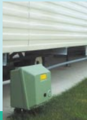
Typical regulator module in ABS kiosk
