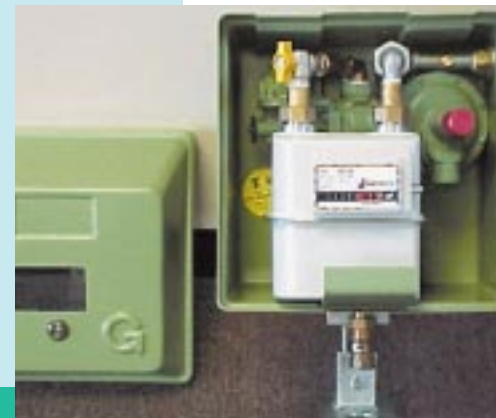
Typical meter module in ABS kiosk with viewing window
