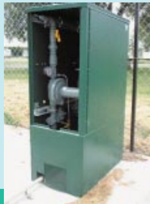
Typical twin stream 1 st stage pressure reduction module.
