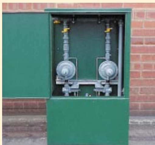
10 million Btu/h twin-stream PRS in kiosk
