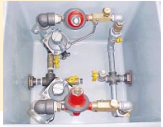
1 million Btu/h twin-stream PRS in pit
