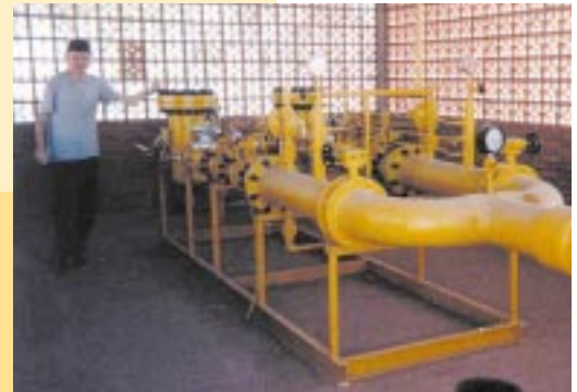
A station in Queretaro
