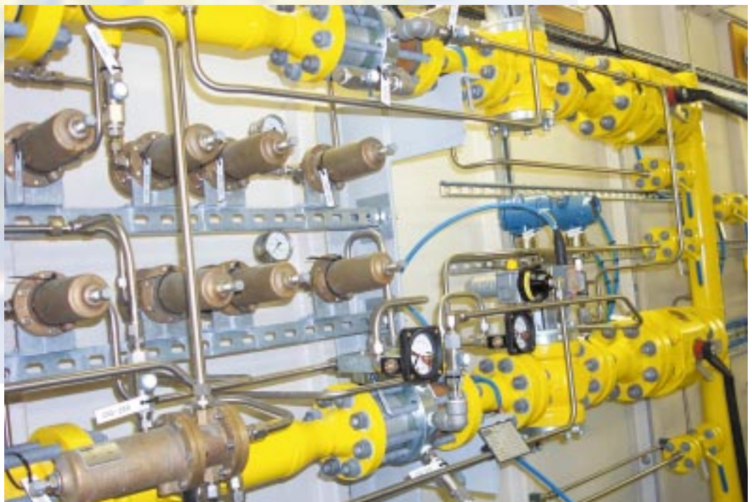
Inside view of the kiosk showing part of the pressure regulation and metering streams
