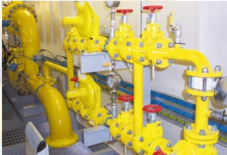
The boiler fuel gas supply
