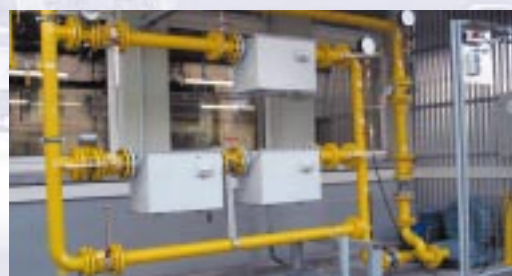
Fig. 4: ELSTER test bench, pressure up to 16 bar, test medium natural gas
