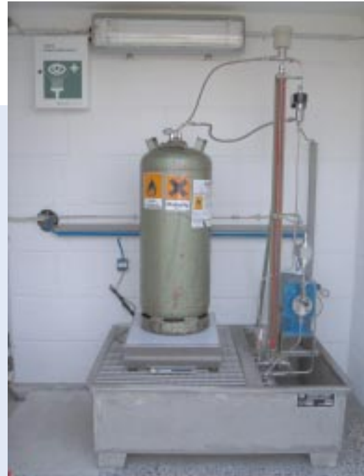
Fig. 1: Odorization system with a weighed 45kg bottle container
