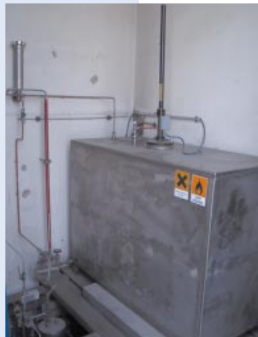
Fig. 2: Medium-sized odorization system with an 800 litre tank. The level is monitored by a magnetic flap.
