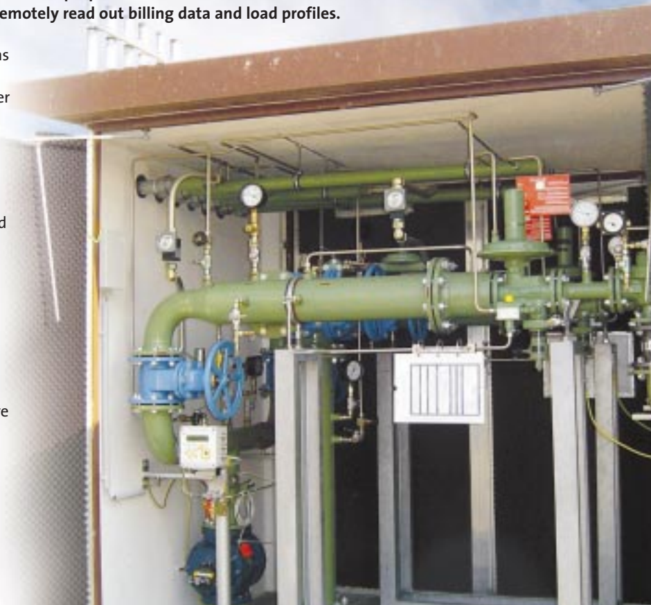
Fig. 2: Gas station without mains supply
