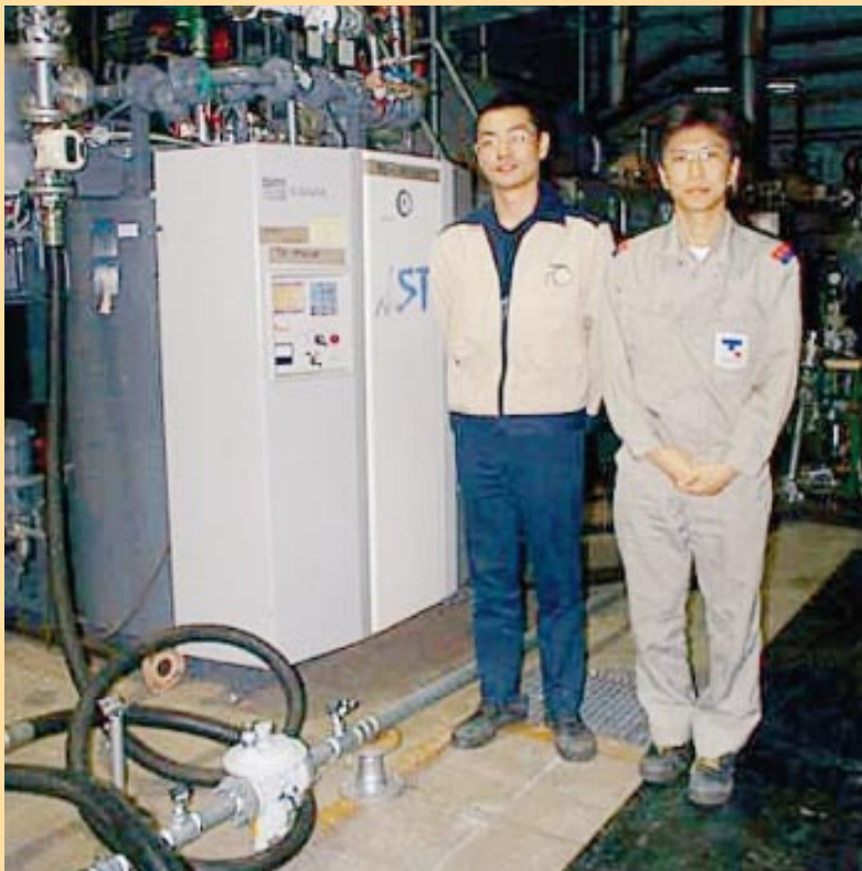
Test bench in a major gas company
