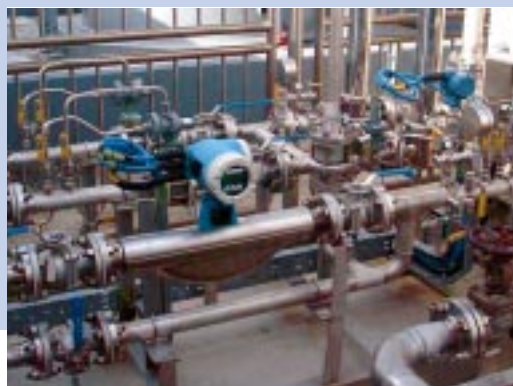
Fig. 3: Equipped with measuring and monitoring instruments
