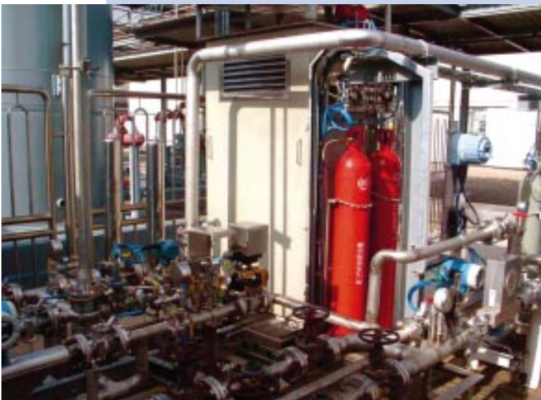
Fig. 2: View of metering and regulation station
