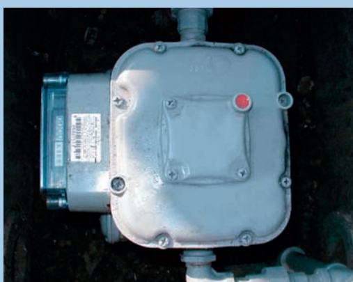
The new Curb Meter with AMR
