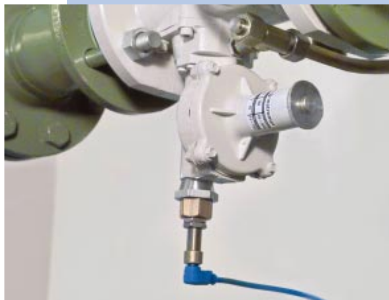
Gas pressure regulator including SSV remote indicator
