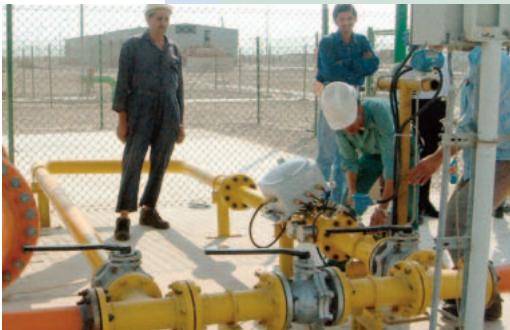
Fig. 2: New U-shaped metering platform for the use of a 4" Q.Sonic USM
