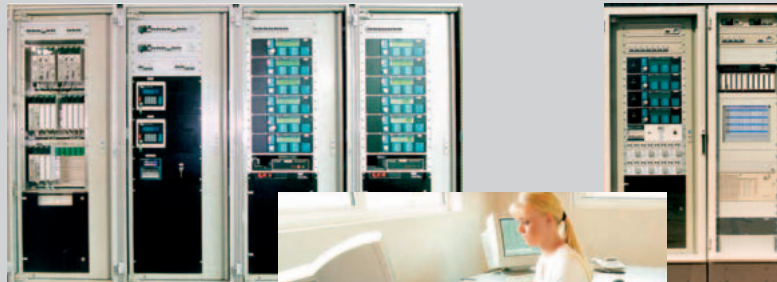
Gas transmission stations
