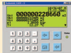
Tele-control panel for the gas-net devices
