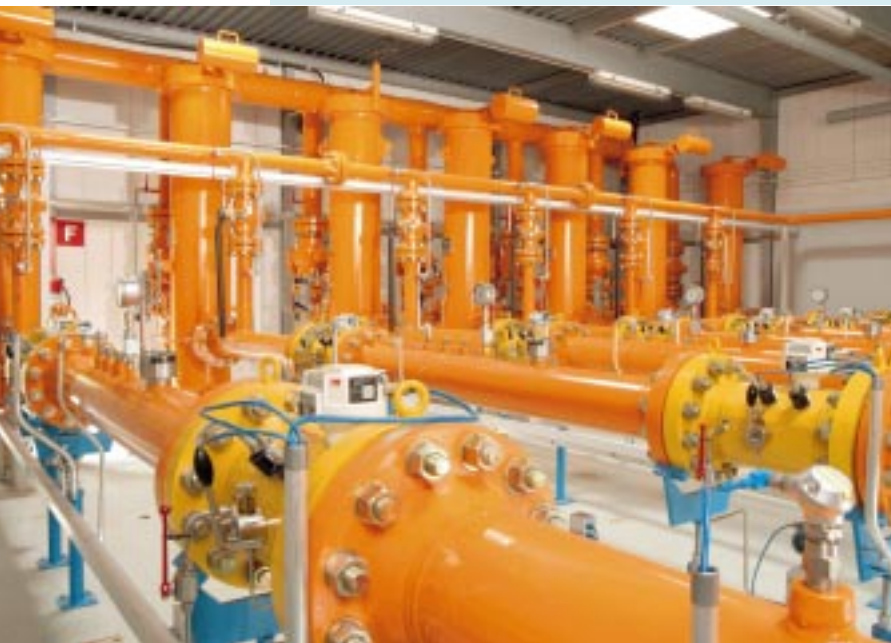
View of the gas measurement room
