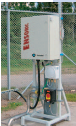
Fig. 2: EnSonic installed in the field
