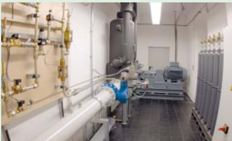
Fig. 3: Machine room with the high-pressure fan
