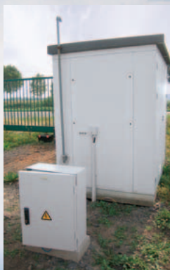
Fig. 1: The electrical cabinet installed near the gas stations, outside hazardous area
