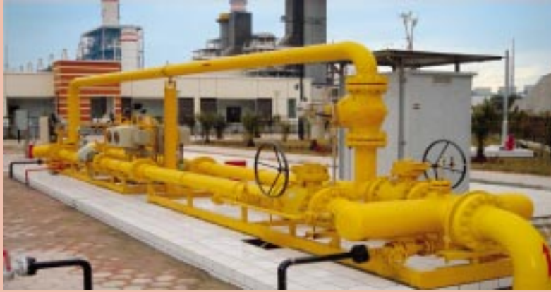
Fig. 1: Hongwan Power Plant station
