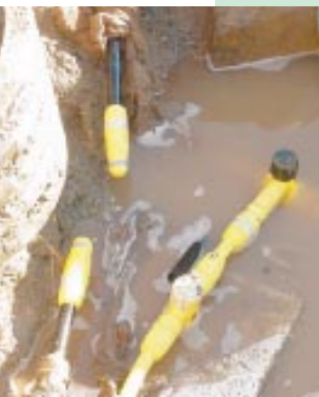
Despite wet weather conditions and temperatures of 2°C, installation of a U-gauge on the basement piping of a commercial building was completed without interrupting the gas supply or causing a drop in pressure
