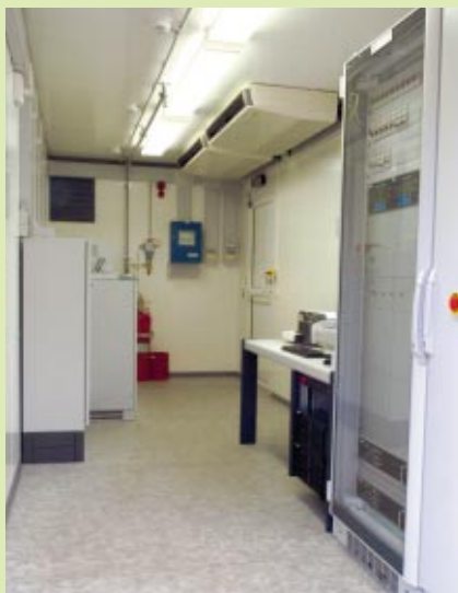
Control shelter (inside)
