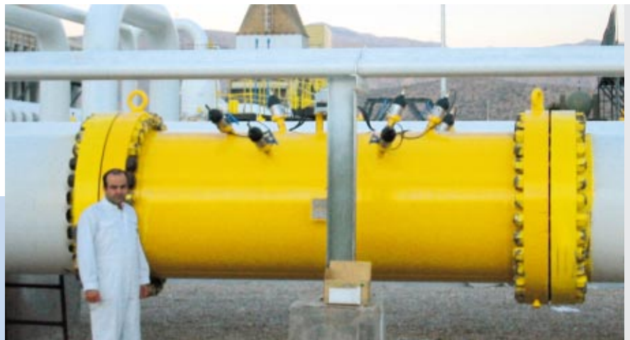
48" ANSI 600 ultrasonic meter in operation in Iran
