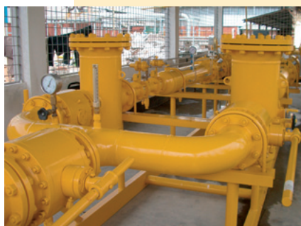
Fig. 1: Natural gas station of a sugar refinery
