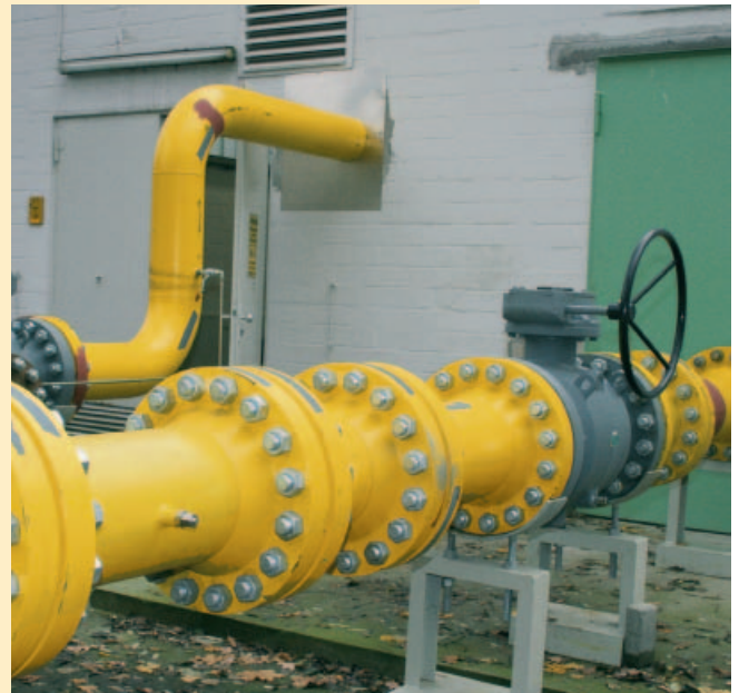
DN 200 pipe sections have become DN 250 pipe sections
