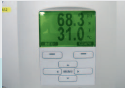
On-site temperature and humidity
