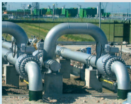
Overview Minerbio plant
