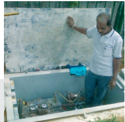
PowerGas operator commissioning the Orpheus 4 module
