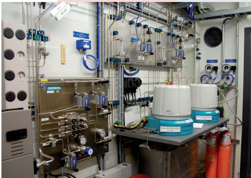
EnCal 3000 in a redundant setup installed in an air-conditioned analyser room
