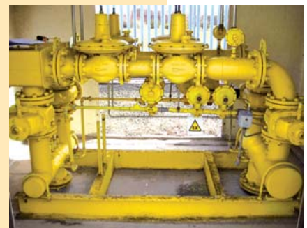
Existing MP/LP district pressure reduction station
