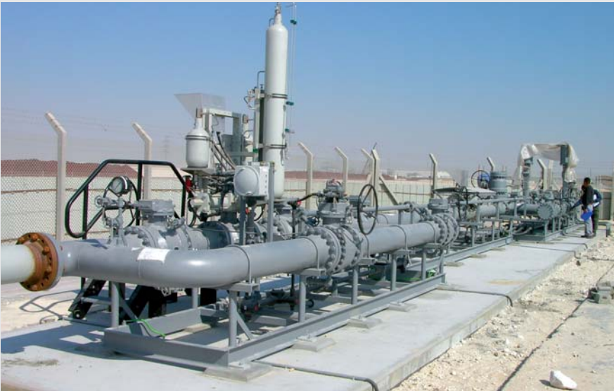
High pressure station installed and prepared for commissioning
