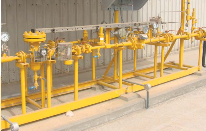
A typical industrial station including emergency shut down, filtration, regulation and metering section
