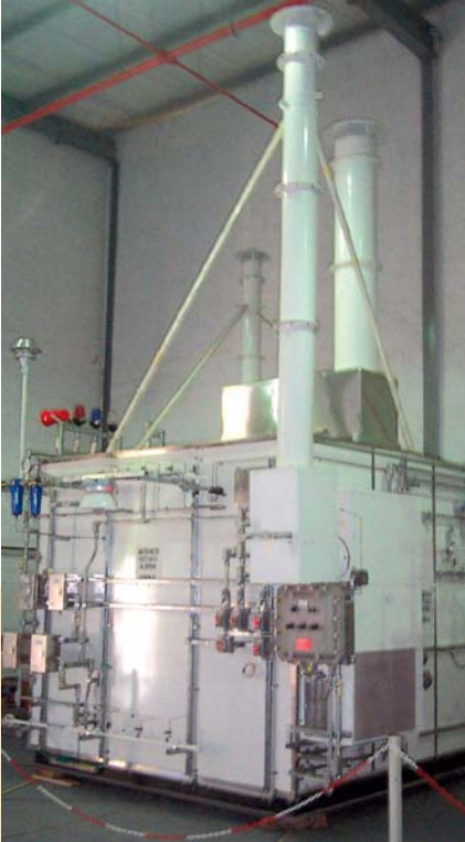
Conditioned analyzer shelter
