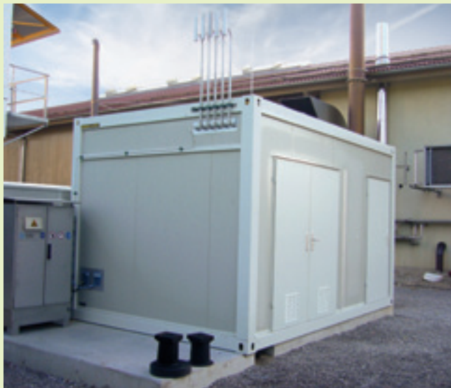
Fig. 3: Container with the biogas injection conditioning, odorizing and official volumetric metering and gas quality analysis
