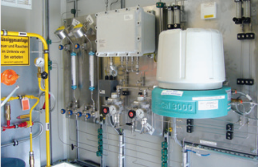
Fig. 6: Gas quality analysis system with test gas conditioning for 2 measured gas streams, gas-lab Q1 and EnCal 3000 for biogas (from left to right)
