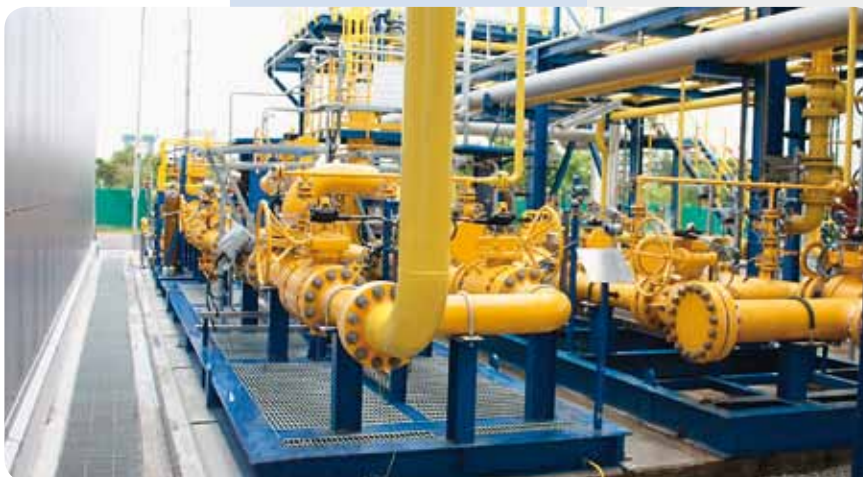
Back view – skid outlet
