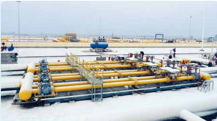
Western part of WEPP II
