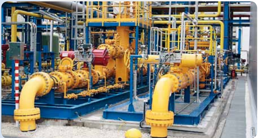
Front view – skid inlet
