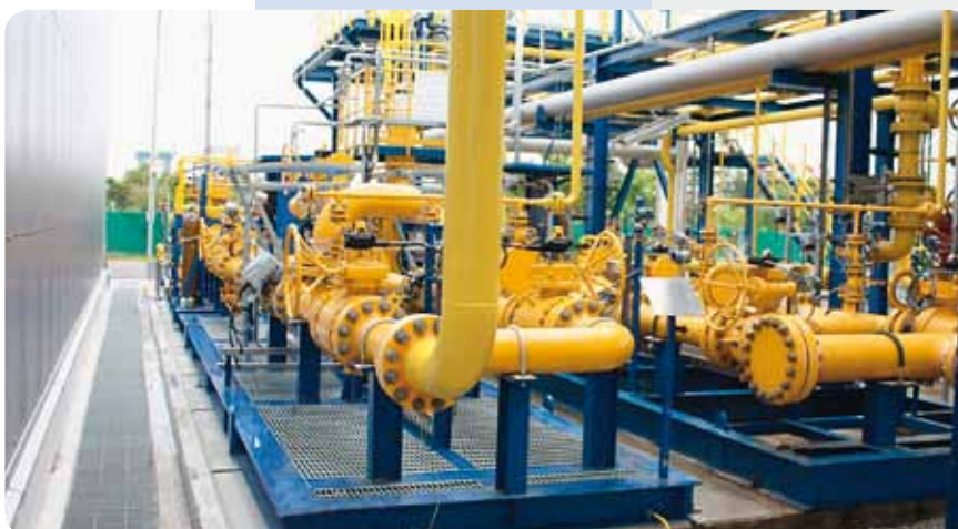
Back view – skid outlet
